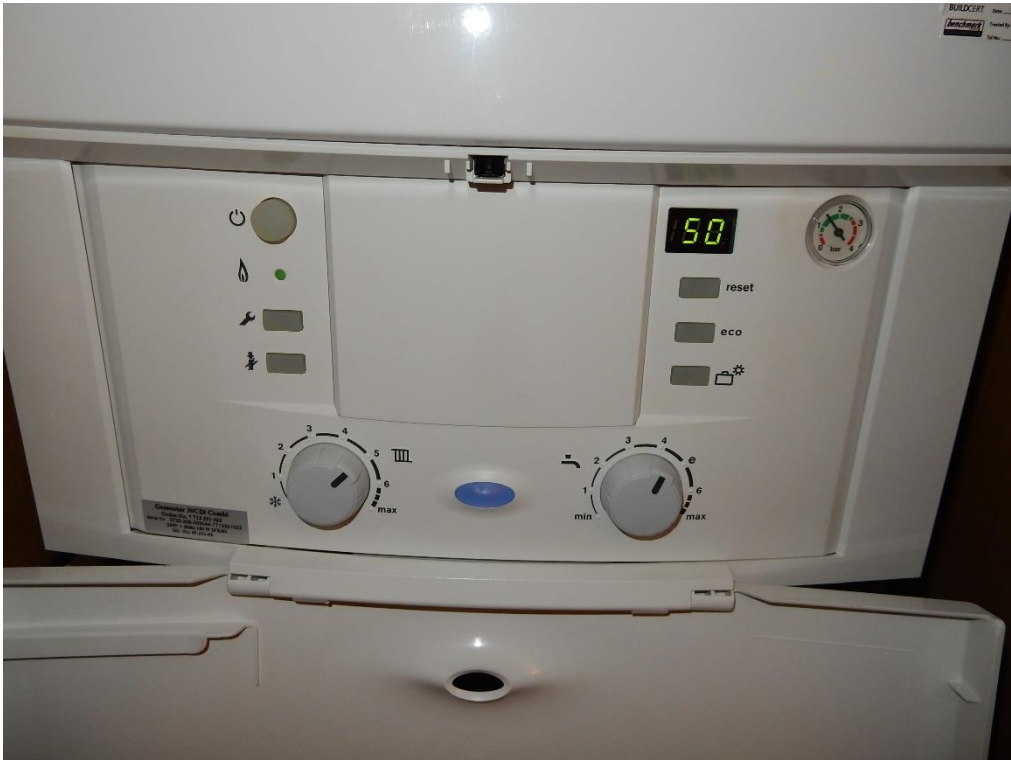
Photo 2 Boiler Control Panel
