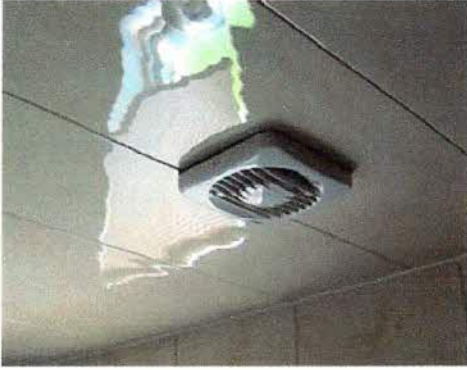
Extractor in bathroom
